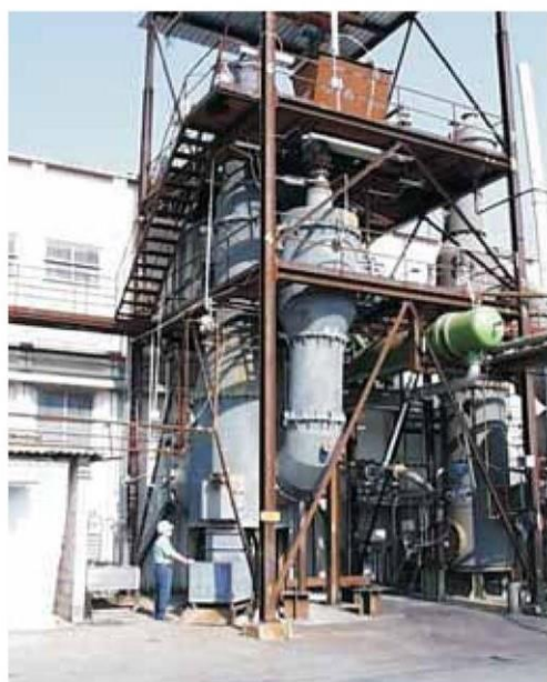
Gasification pilot plant (400 kg/h)
